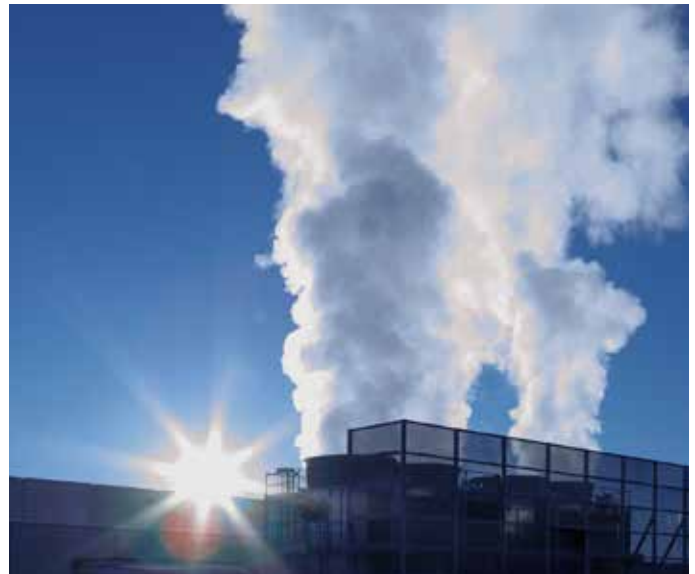
▲ Completed in May 2020, the Exascale-Class Computer Cooling Equipment project increased the existing water-cooling capability at the Laboratory's Strategic Computing Complex, where the new supercomputer, Crossroads, will reside. Crossroads is due at the Laboratory in 2022.
