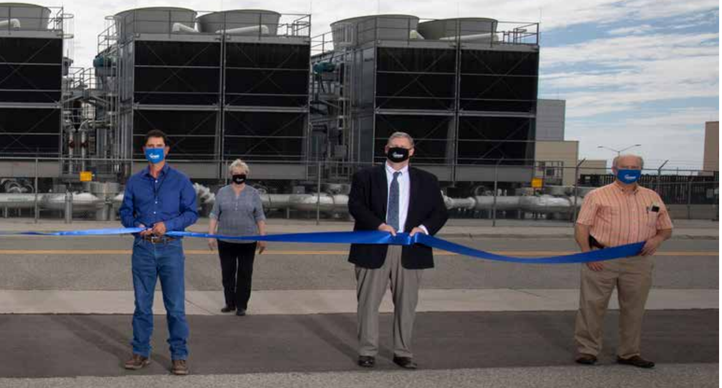
◆ From left: John Sarrao, Thom Mason, Gabriela Lopez-Escobedo, Lisa Gordon-Hagerty, John Gallegos, Kathye Segala, Michael Weis, and Gary Grider cut the ribbon in front of the new cooling towers at the Laboratory's Nicholas C. Metropolis Center for Modeling and Simulation on July 16.
